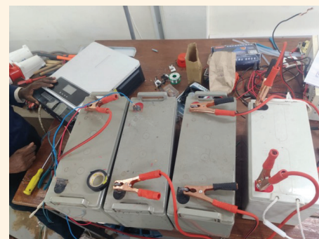
Figure 20: Batteries storing solar energy for use when solar lights are off
